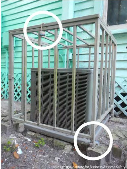
A steel cage around ground-mounted air conditioning units can prevent theft as long as it's bolted to the ground and locks are used, which are circled above.
