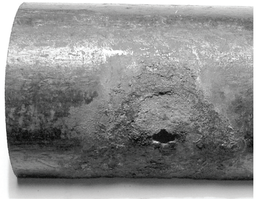
Photo courtesy of National Fire Protection Association
