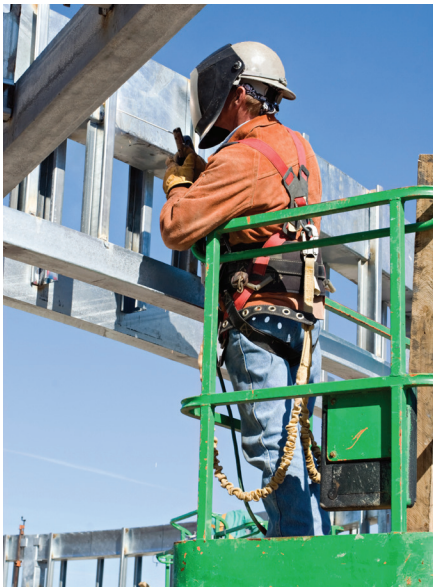
Aerial lift with full guardrails.
