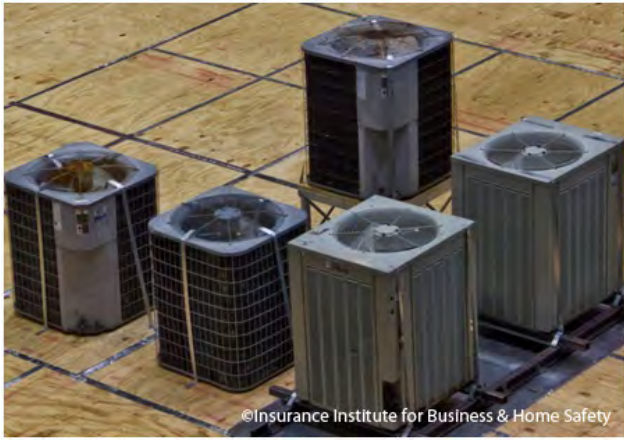
Secure AC units like those shown above in order to reduce the risk of damage to the equipment during high winds.
