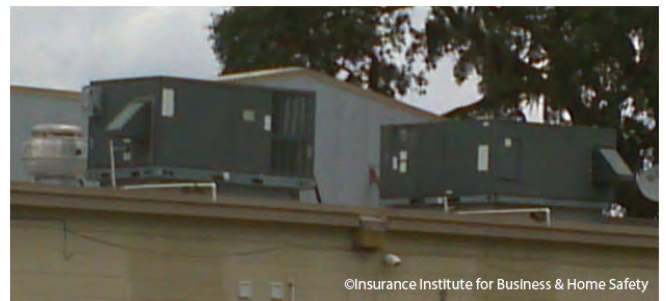
Regular inspection of commercial rooftop equipment, as shown above, is critical in preventing significant damage during severe weather.
