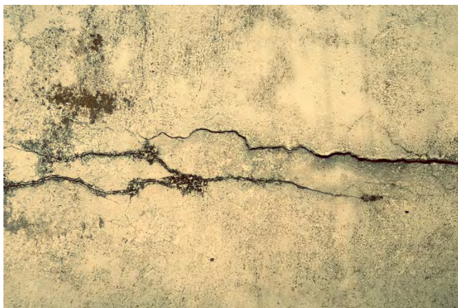
Inspect your walls for cracks caused by water damage, as shown above.
