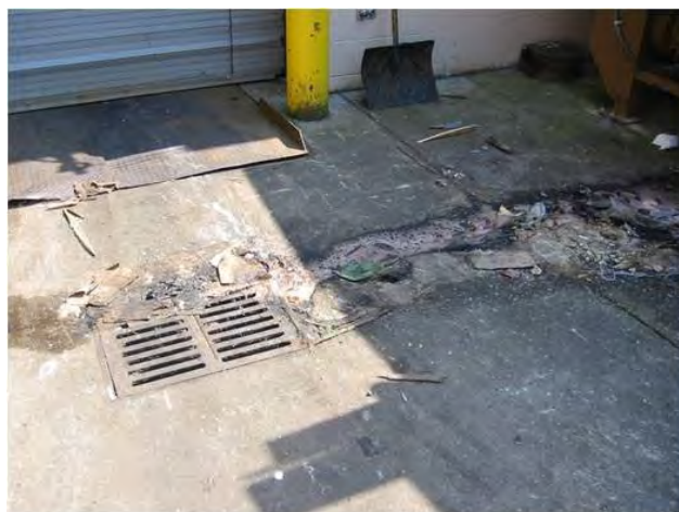
Debris can clog exterior drains like the one shown above, and possibly result in water damage.
