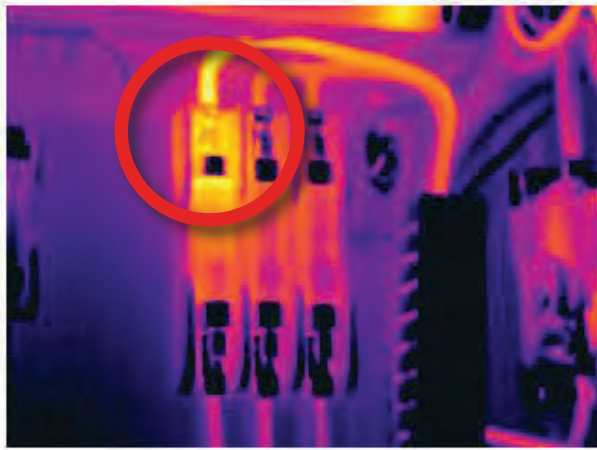
Shown above is an example of what a hand-held thermal scanner could show you, with a potential hot spot circled.
