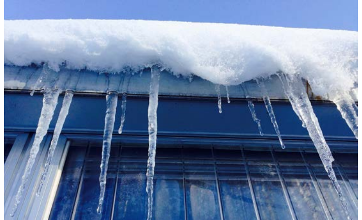
Don't let debris, dirt and leaves collect in gutters and downspouts; this can lead to damaging ice dams and heavy snow buildup.
