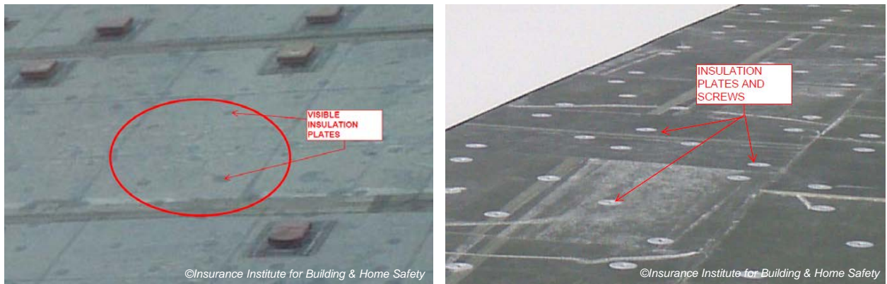
Figure 2. Adhered EPDM with insulation plates (left) and TPO cover removed exposing insulation plates (right).
