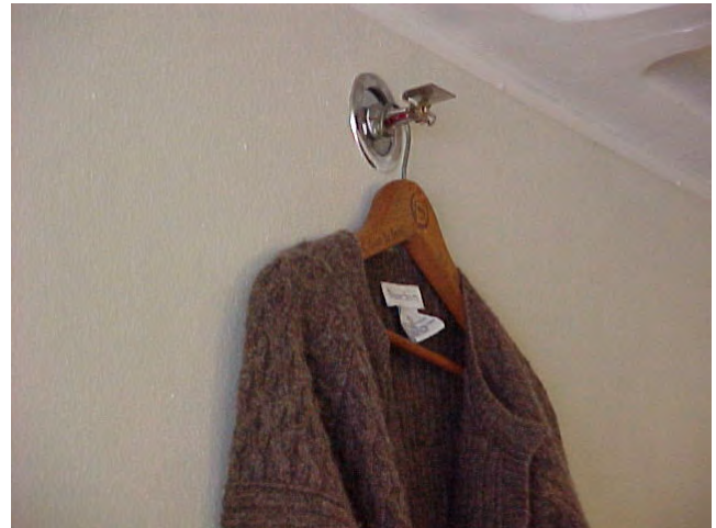
The picture above is an example of what NOT to do. Never use a sprinkler head as a clothing hook.
