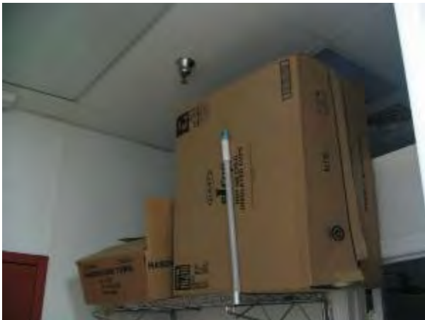
Make sure all fire sprinkler heads are not blocked in any way. This photo shows boxes that are too close to the sprinkler head. This may prevent heat from reaching the head and it can reduce the water spray pattern.
