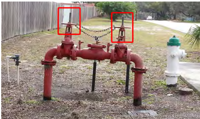
A backflow preventer with two outside screw and yoke (OS&Y) valves is in the open position since the valve stem is visible (highlighted by red boxes). When an OS&Y valve is shut, the stem is not visible.
