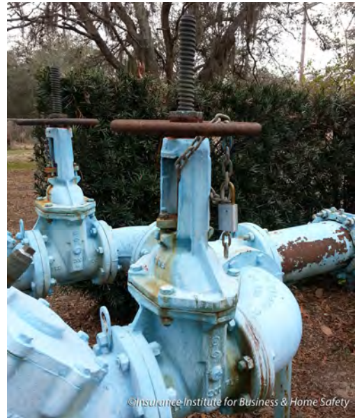
The lock and chain on the backflow preventer pictured above indicates that it is in a locked position.
