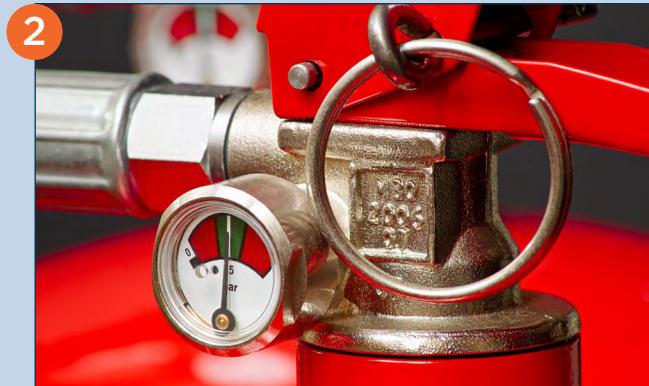
2 Monthly Inspection: Ensure That All Extinguisher Tanks Are Full
