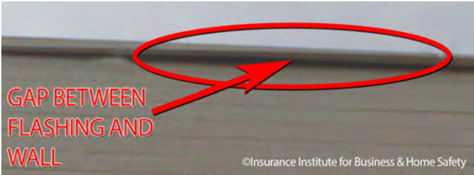
Look for gaps between the flashing and the wall when inspecting edge flashing.
