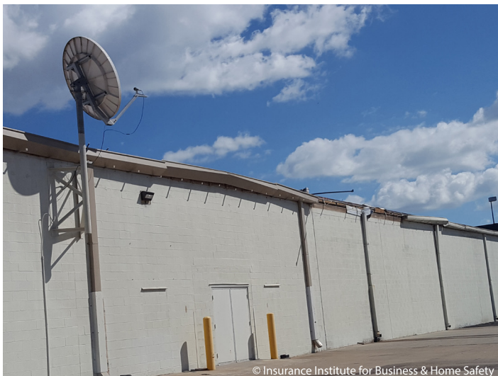
Gutter damage in Texas after Hurricane Harvey.
