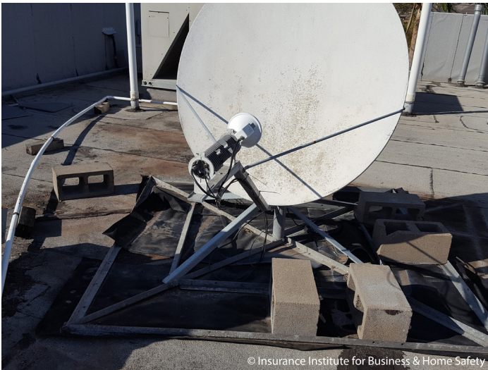
Satellite dish damage in Texas after Hurricane Harvey.
