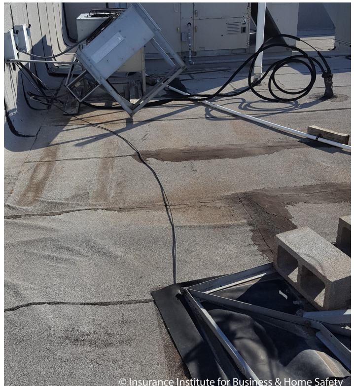
Roof-mounted equipment damage in Texas after Hurricane Harvey.
