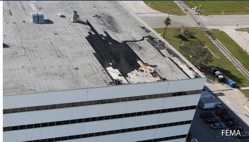
Roof damage caused by Hurricane Matthew in 2016.
