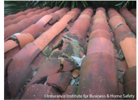
The tiles on this roof are damaged and should be replaced.
