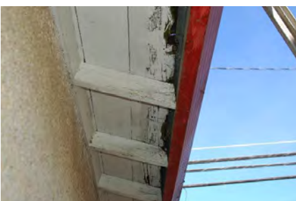
Decayed wood at the roof edge—more readily ignited from any flaming exposure resulting from burning debris in the gutter. Source: Stephen L. Quarles
