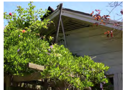
Vegetation growing over a trellis structure. If ignited, flames would impinge on the side of the house, including the nearby gable end vent. Source: Stephen L. Quarles
