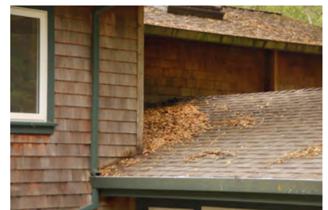
Replacing siding "locally," in areas where it meets the roof on a complex roof design, such as that shown here, would be more affordable than "global" replacement. Source: Stephen L. Quarles
