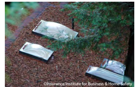
Flat (top photo) and domed (bottom photo) skylights. Note propensity for debris to accumulate on top of flat versus domed skylights.
